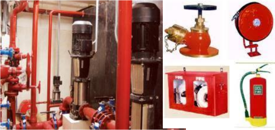
Fire fighting facility
